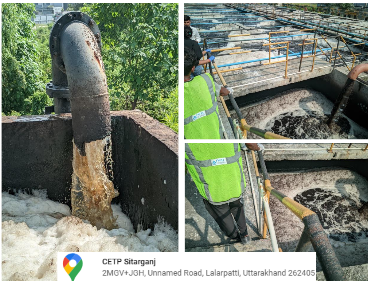
1.2.e SIDCUL Treatment Plant
