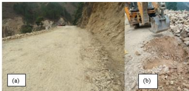
(a) View of Site before laying of premix carpet (b) collection soil and gravel from the existing pavement
