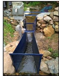
e) Parshall flume at stream
