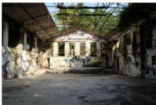
Damaged sheet roof of the yoga hall
