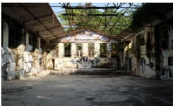
Damaged sheet roof of the yoga hall
