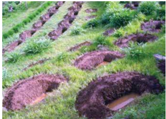
Springshed trenches complemented by vegetative measures were part of Dhara Vikas Programme of RM&DD in Sikkim State.
